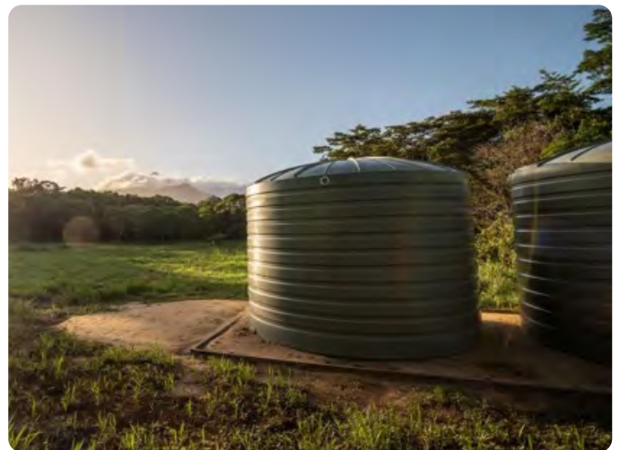
The newly installed water tanks. Image: © Martin Stringer
