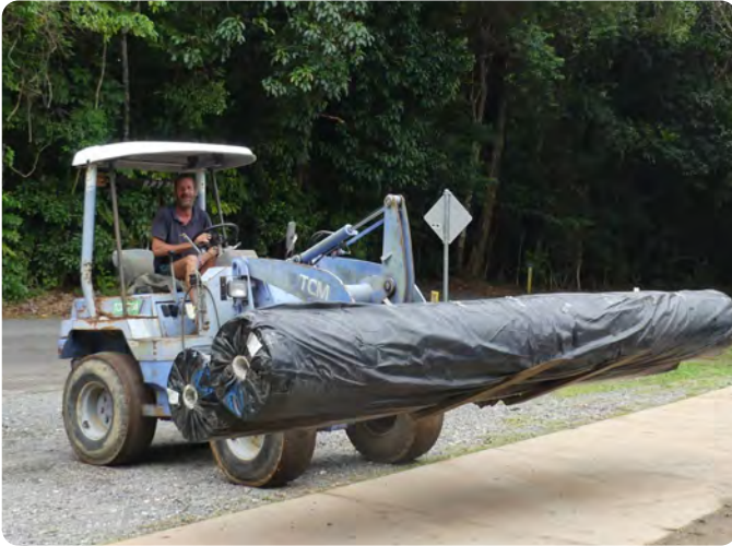
Greg moving the last couple of rolls of Geofabric for the shade house - it's very heavy! Image: Barbara Maslen
