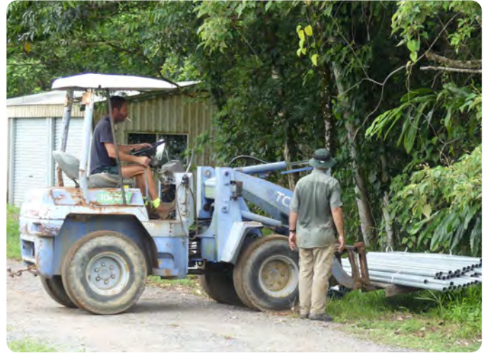
Unloading some of the steel posts for the shade and propagation houses. Image: Barbara Maslen
